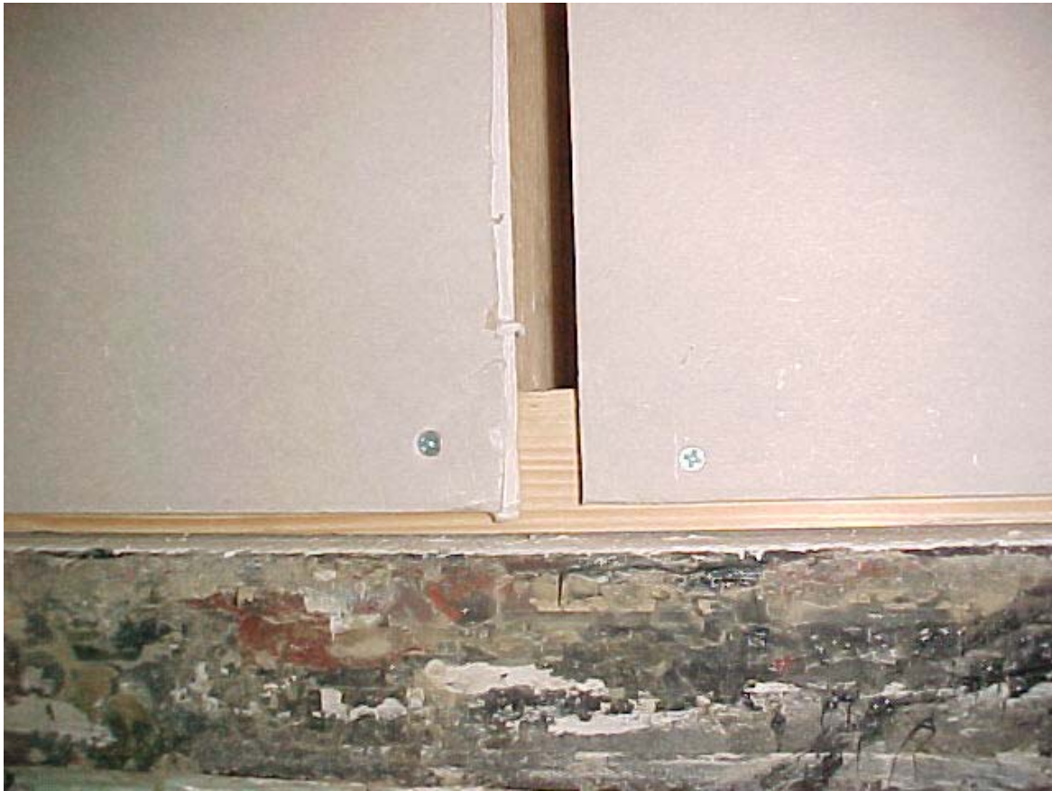
Photograph 2: Unsealed Partition Close-Up
